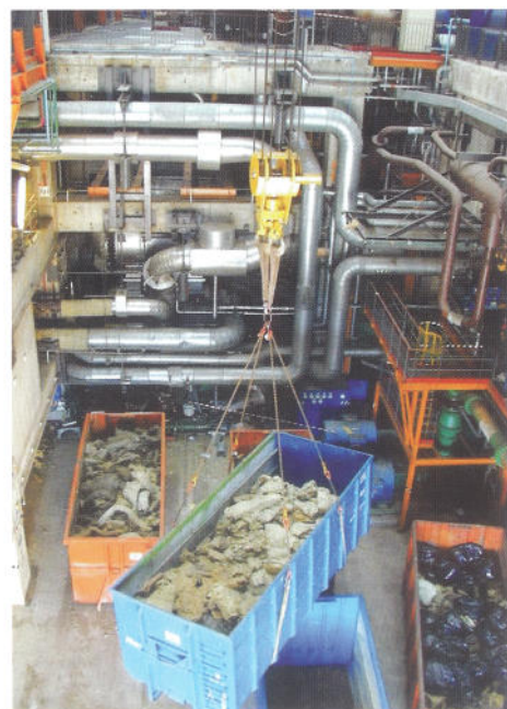
Removing insulation waste. The tangle of pipework is visible in the background.
