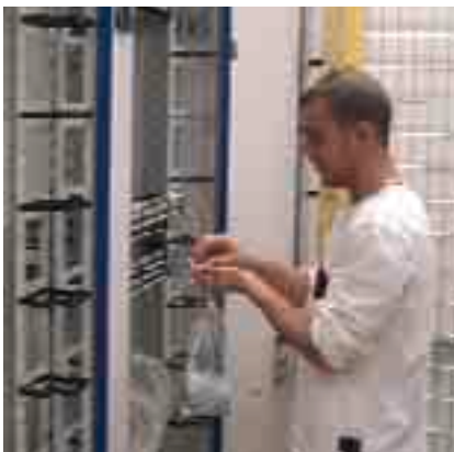
Connecting one of the 120,000 RJ 45 connectors at the site.
