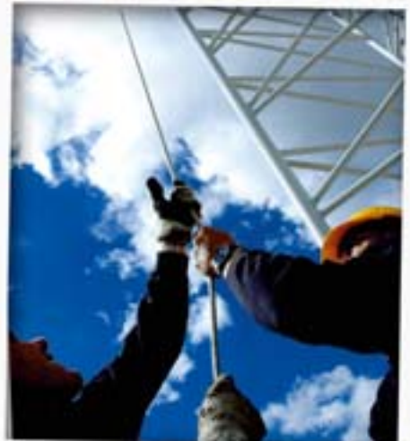
TONNIE AND ROB HOIST THE ANTENNA TO THE TOP OF THE PYLON, WHERE IT WILL BE COLLECTED BY JOHNNY AND DANNY AND MOUNTED ACCORDING TO THE SPECIFICATIONS IN ORDER TO ENSURE THE BEST NETWORK COVERAGE.
