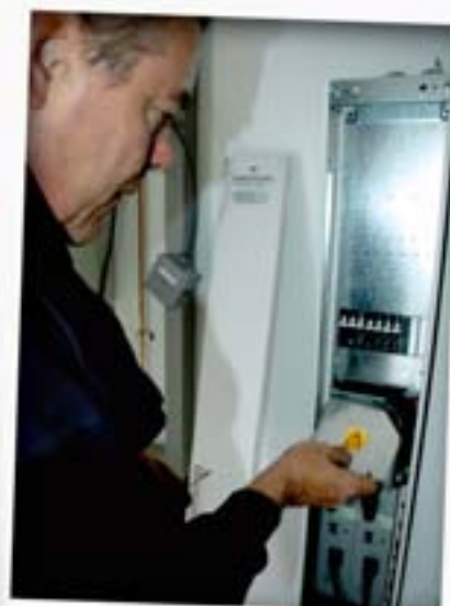
ROB INSTALLS AN ANTENNA CONNECTION RACK IN THE CABINET.
