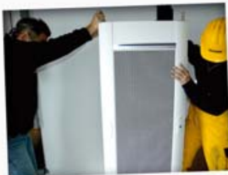
IN THE TELECOM BUILDING, ROB AND EELCO INSTALL THE RACK IN WHICH THE HARDWARE COMPONENTS ARE TO BE FITTED.
