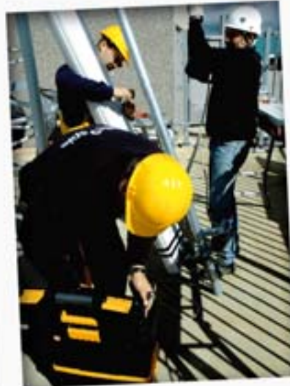
TONNIE IN THE FOREGROUND, ROB DE FEY (TELECOM TECHNICIAN, RIGHT) AND EELCO, ARE READYING THE ANTENNA FOR INSTALLATION. THEY COVER THE ENDS OF THE ANTENNA CONSTRUCTION. THIS AVOIDS NOISE PROBLEMS SUCH AS WIND IN THE TUBES. SIX ANTENNAS WILL BE FITTED TO THE TOP OF THIS PYLON. (3x GSM AND 3x UMTS)
