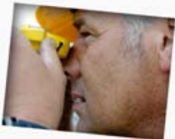
AFTER SUPERVISING THE OPERATION, TONNIE VERIFIES ROUGHLY THE ORIENTATION OF THE ANTENNA WITH RESPECT TO THE GEOGRAPHICAL COORDINATES CALCULATED DURING THE PRELIMINARY STUDIES. THE ORIENTATION OF THE ANTENNAS WILL BE TUNED WITH A GPS SYSTEM.
