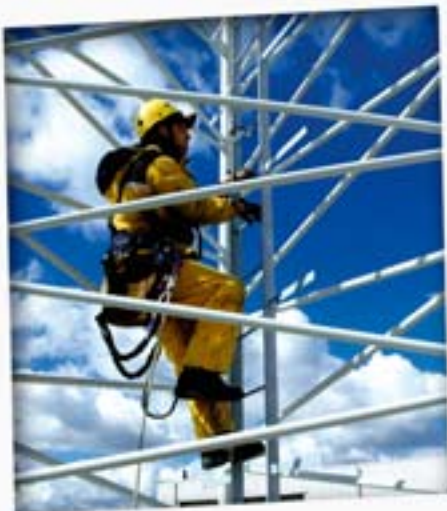
DANNY PAP (TECHNICIAN) CLIMBS TO THE TOP OF THE PYLON TAKING WITH HIM A ROPE. A PULLEY WILL BE INSTALLED IN THE TOP OF THE MAST SO THAT THE ANTENNAS AND ALL THE EQUIPMENT NEEDED FOR CONNECTION CAN BE HOISTED UP.
