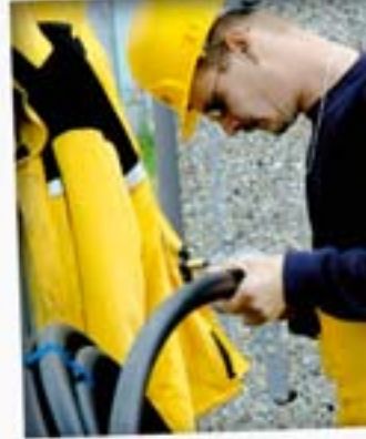
THE CONNECTION CABLES MUST BE THEY ARE HOISTED TO THE TOP OF DE VOOGT (TECHNICIAN) INSERTS THE END OF ONE OF THE CABLES. OF CABLES WILL BE NEEDED FOR INSTALLED ON THE PYLON.
