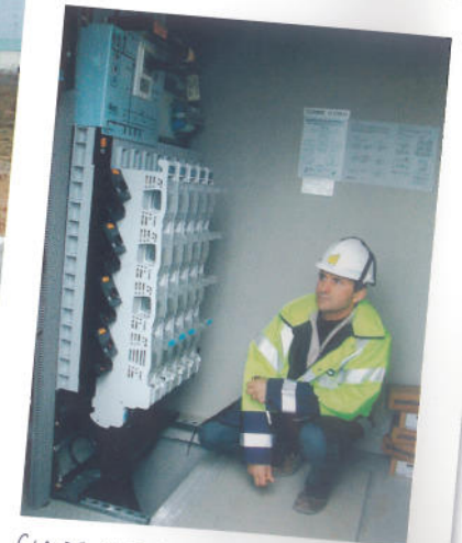
CLAUDE IN THE LOW-VOLTAGE CABLE CONNECTION SUBSTATION.
