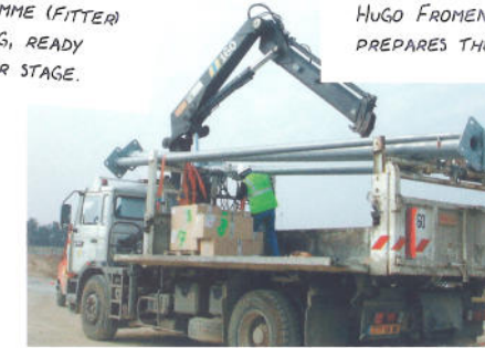
CHRISTIAN PONSARD (DRIVER) UNLOADS THE LAMP UNITS AND LAMP-POSTS AT THE SITE.
