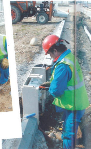
SERGE WIRES UP THE FALSE DISCONNECT CABINET THAT WILL BE USED TO POWER THE DIFFERENT LOTS INSTALLED IN THE AREA.
