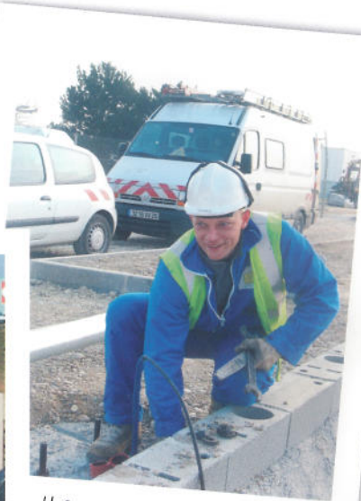
HUGO ADJUSTS THE BOLTS THAT WILL BE USED TO ANCHOR THE LAMP-POST.
