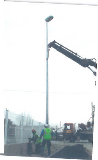
THE 8 M TALL LAMP-POST IS RAISED INTO POSITION. SERGE VERNET (FOREMAN) BOLTS IT IN PLACE.
