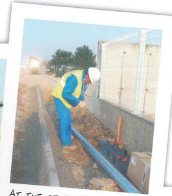
AT THE OTHER END OF THE DUCT, NOËL DELHOMME (FITTER) CATCHES THE STRING, READY FOR USE AT A LATER STAGE.
