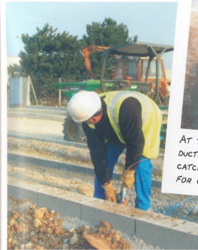
JACQUES FUMAT (FOREMAN) USES COMPRESSED AIR TO BLOW A LENGTH OF STRING ALONG A DUCT. THIS STRING WILL SUBSEQUENTLY BE TIED TO THE ELECTRIC CABLE AND USED TO PULL IT THROUGH THE DUCT.
