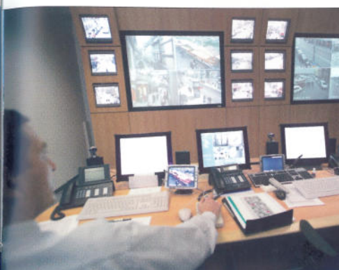
Left: a Strasbourg City Council operator at their workstation in the video surveillance control centre.
