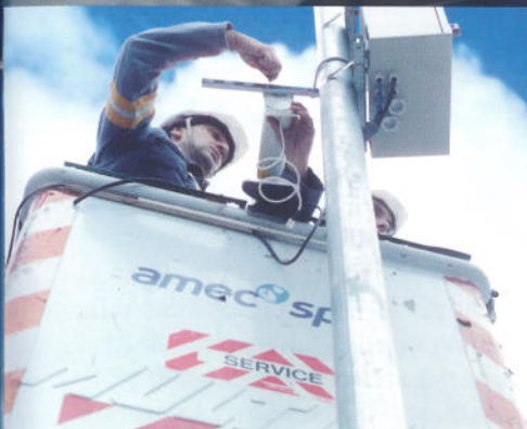
Above: Philippe Schwarz sets up the WiFi receiver. The photos on the left-hand page and opposite: show Philippe Schwarz installing the cameras.
